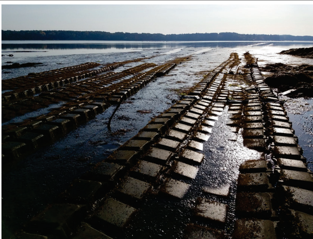
Figure 3. SRP western tidal flats with concrete mattresses at spring low tide on October 19, 2020. Note the shallow trenches of the buried cables visible beyond the mattresses.
